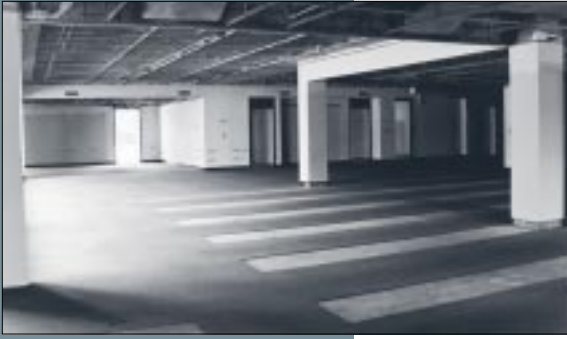
Marquand Library stripped of its books and shelving, ready for construction to begin
