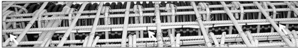
Figure A.4. Sensors AB 2 and AB 3 before pouring of concrete; anchoring points are indicated with arrows.
