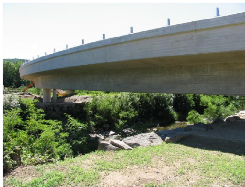
Figure 23 View to main span of Ricciolo Viaduct (see online version for colours)
