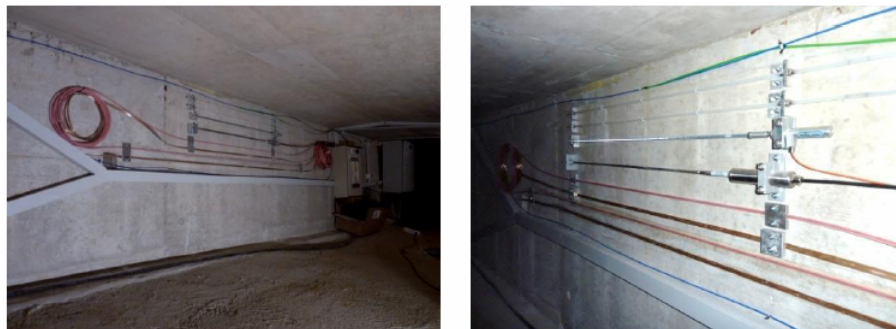
Figure 15 General views of the long-gauge deformation sensors installed on Ricciolo Viaduct for assessment of their performance in real field conditions (see online version for colours)
