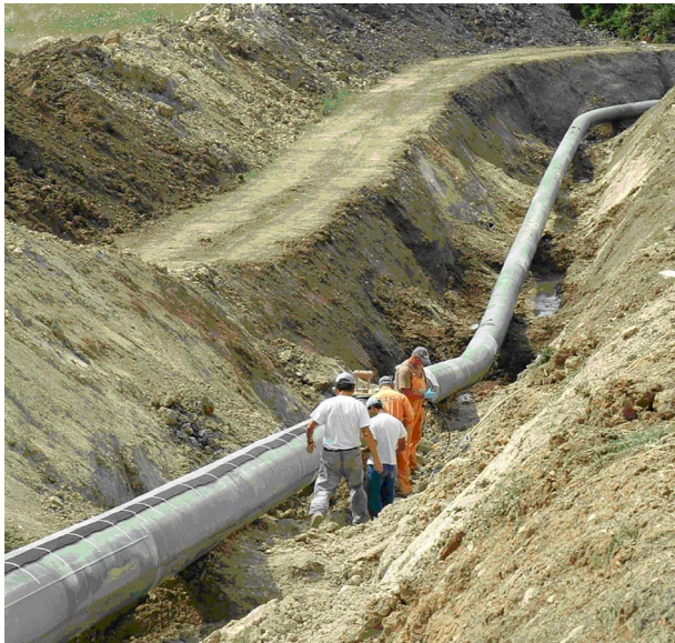
Fig. 8 SMARTape on the gas pipeline
