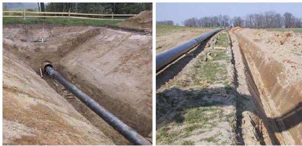
Fig. 6 Construction phase of a buried brine pipeline in the north-east area of Berlin. The fiber optics cable is placed in the sand at the 6 o'clock position about 10 cm underneath the pipeline [4].
