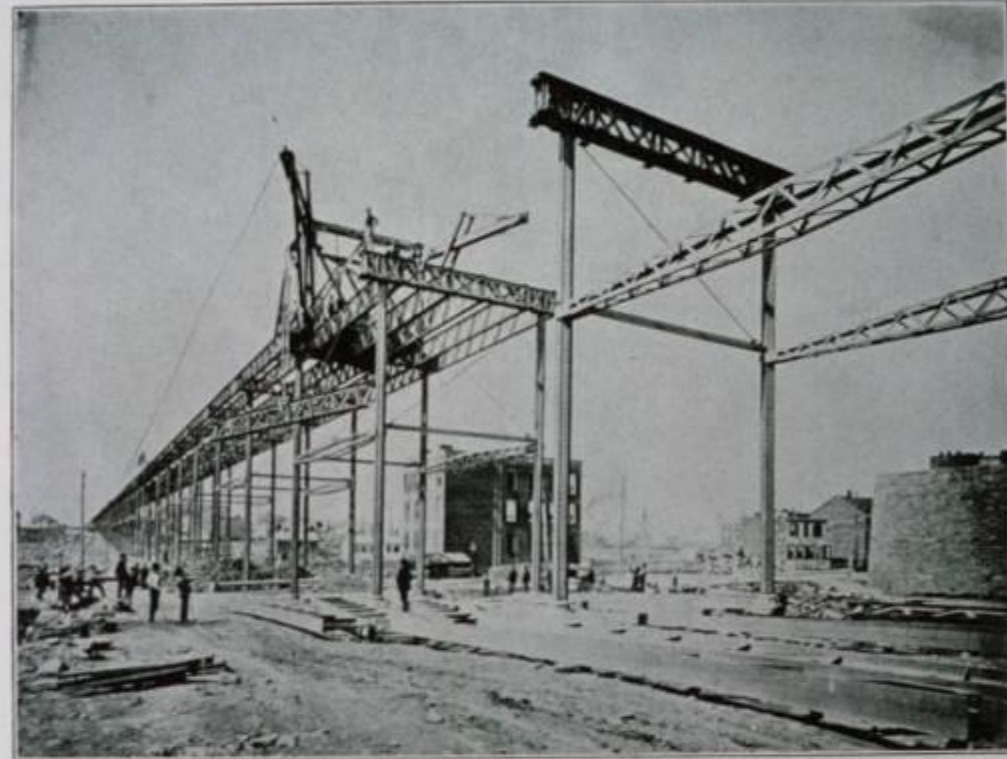
STRUCTURE OF THE METROPOLITAN ELEVATED RAILWAY COMPANY (SIXTH AVENUE LINE) BEING ERRECTED ON NINTH AVENUE (COLUMBUS AVENUE) IN 1878-79
