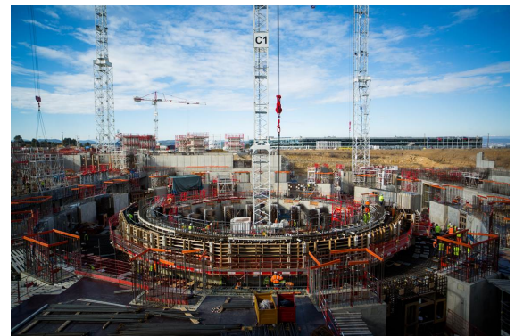
Figure 6.2: After years of delay and continued uncertainty in cost and timeline, ITER construction has begun. The circular structure is the beginning of the building that will house the tokamak. The photo is from February 2016 [16].
