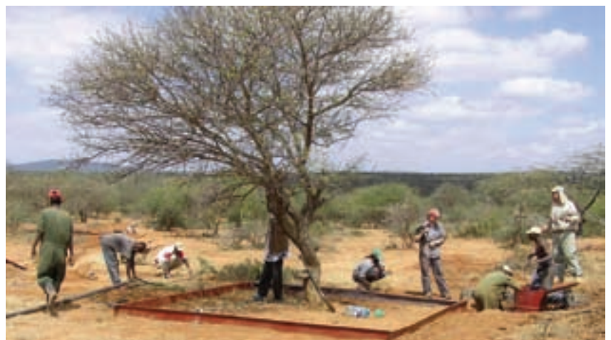
Koiya research scouts, Alex Lester, Trenton Franz, and fundis from Modsan Hardware install rainfall runoff catching equipment and electronic soil moisture probes at Koiya. Runoff is collected inside the walled area, and drains into an underground storage tank where sensors continuously measure the water volume.
