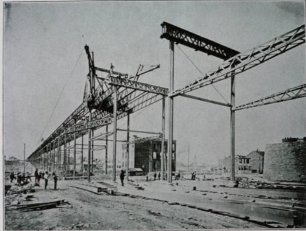
STRUCTURE OF THE METROPOLITAN ELEVATED RAILWAY COMPANY (SIXTH AVENUE LINE) BEING ERECTED ON NINTH AVENUE (COLUMBUS AVENUE) IN 1878-79
