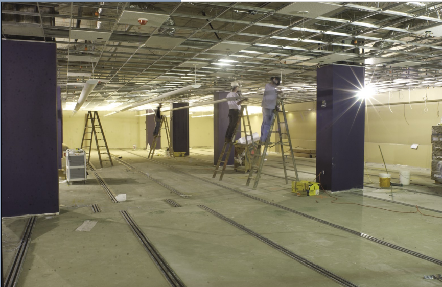
Workers install wiring in the new below-ground book stack and study wing; the tracks for compact book shelving are already in place
