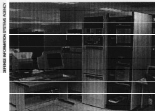
Defense Simulation Internet experimental integration area at the Network Engineering and Assessment Facility Laboratory of the Defense Information Systems Agency's Center for Systems Engineering in Reston, Virginia.
